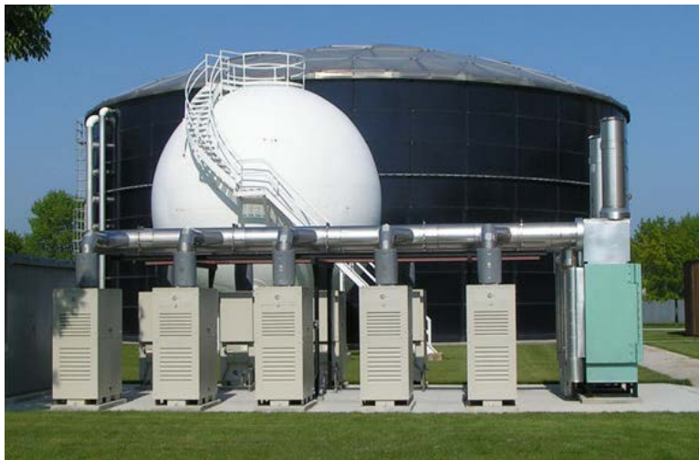
Figure 19: Microturbine Installation at the Sheboygan Regional WWTTP
