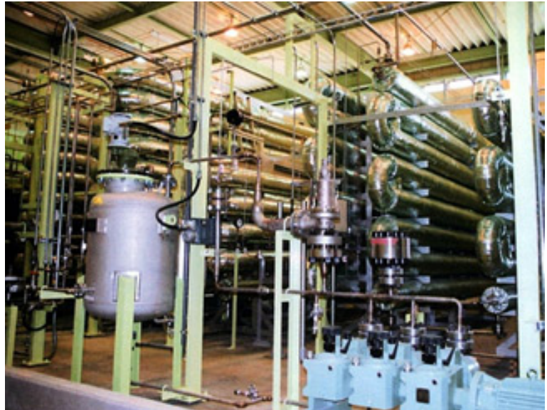
Figure 25: Supercritical Water Oxidation Facility in Cork, Ireland
