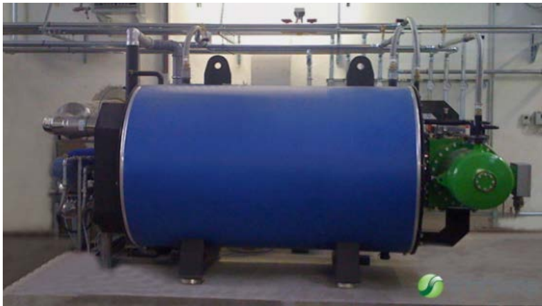
Figure 20: Stirling Engine Installation at the Niederfrohna WRRF in Germany
