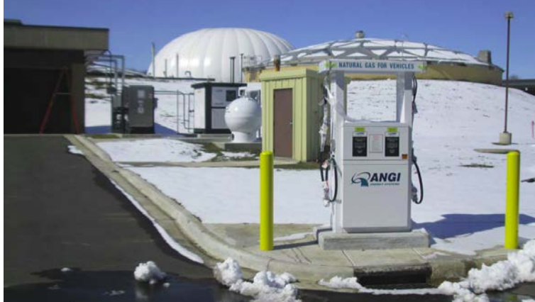
Figure 21: BioCNG installation at Janesville, WI WWTP (BioCNG, 2012)
