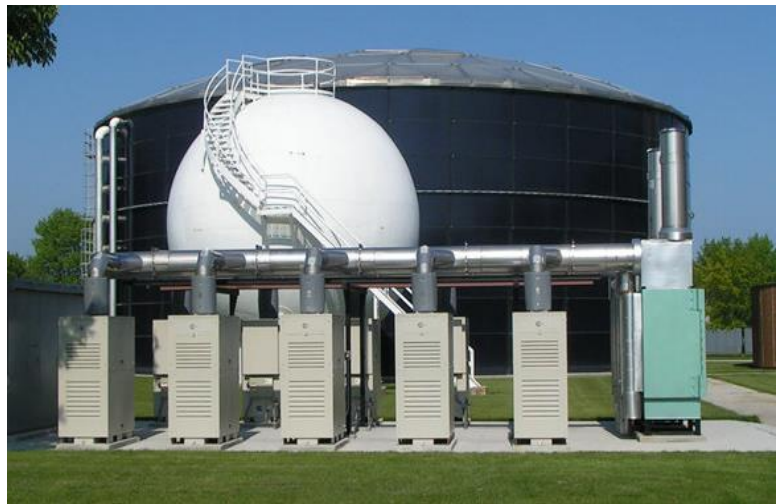
Figure 15: Microturbine installation at the Sheboygan Regional facility
