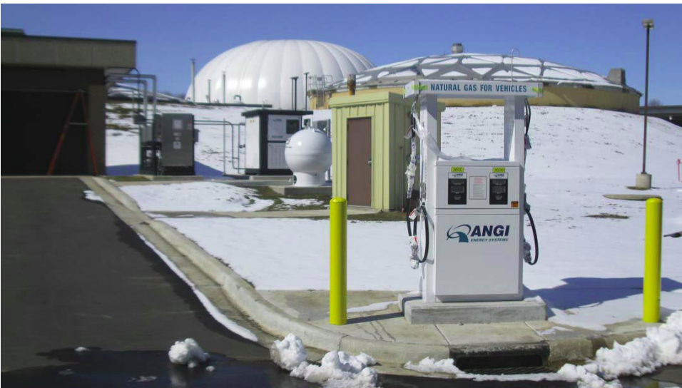
Figure 18: BioCNG installation at Janesville, Wisconsin, facility (BioCNG, 2012)
