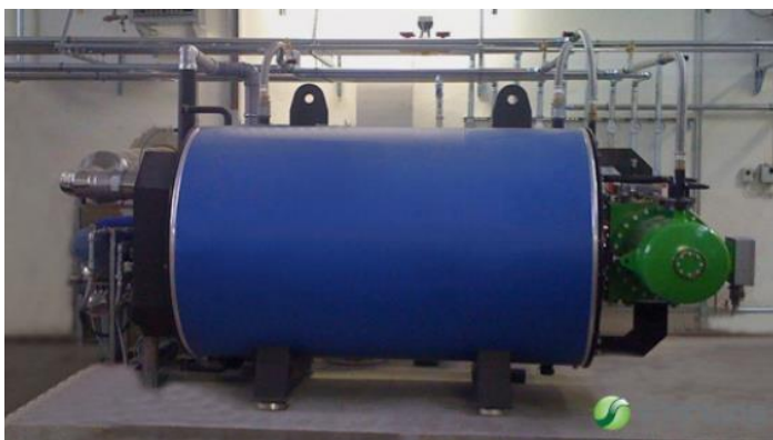
Figure 16: Stirling engine installation at the Niederfrohna facility in Germany
