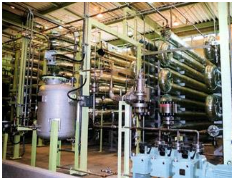
Figure 21: Supercritical water oxidation facility in Cork, Ireland
